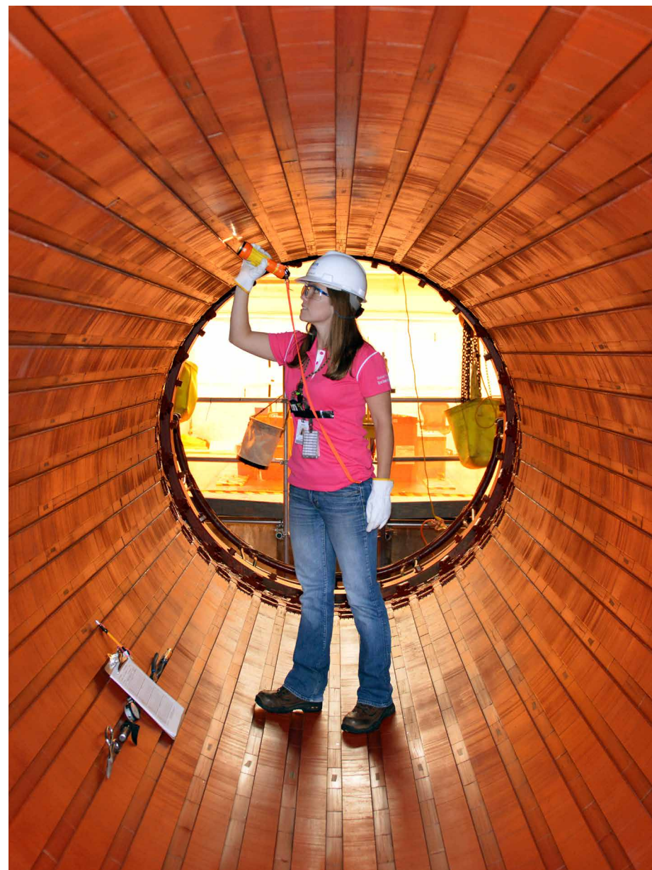
Inspecting power generation equipment at Byron Station.
